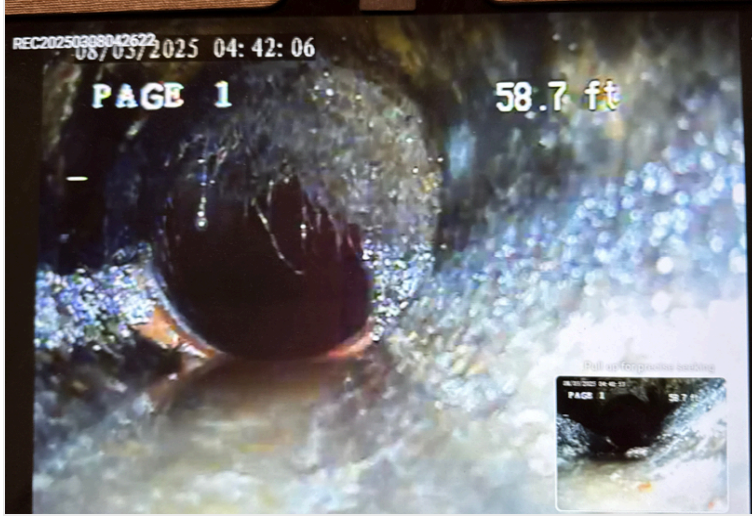
○ Findings @: 58 ft Root Intrusion. Augering.
