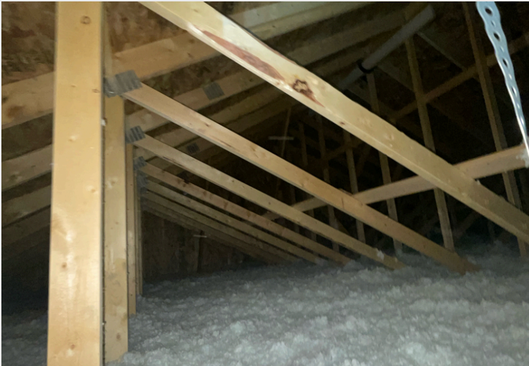
Attic Construction Overall Designed to support the roof with rafters or trusses.
