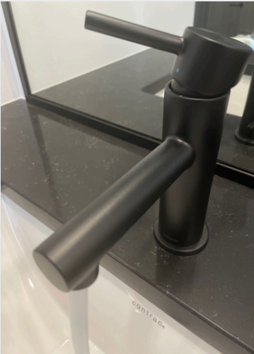
Hot Water Thermal We always thoroughly run ALL plumbing fixtures & check for temperature variance.
